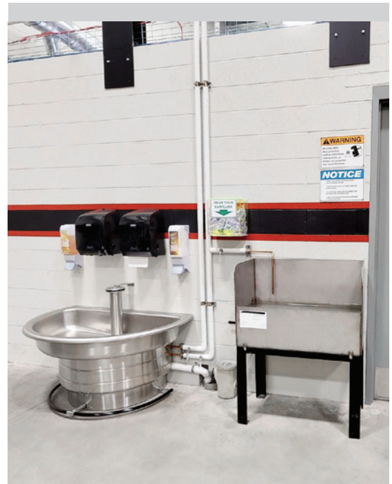
Figure 2-5: Placement of a Quench Tank Near Grinding Stations is Important for Efficiency and Safety. Areas Where Materials are Cut Should be Located With Easy Access by Instructor.
