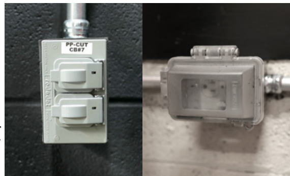
Figure 2-20: To Enhance Safety Within Welding Areas, All Electrical Outlets Should Have Covers.
