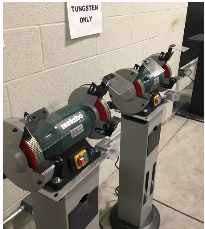
Figure 2-12: The Ideal Grinding Station Offers Easy Access to a Quench Tank with Adequate Dust Control
