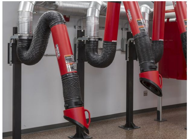
Figure 2-17: Centralized Fume Extraction Arms
