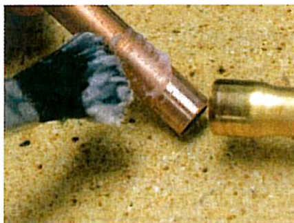
« Image 1. Since flux contains moisture—the enemy of an HVACR system—techs should keep excess flux from inside the lines using a brush to apply a thin coating of the substance to copper tubing.
