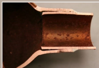
Fig. 2 Sectioned brazed joint showing lack of filler metal penetration
