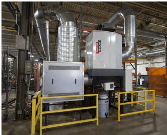
Push/Pull System installed at Elgin Sweeper Company
