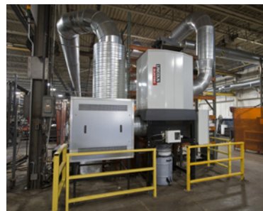
Push/Pull System installed at Elgin Sweeper Company
