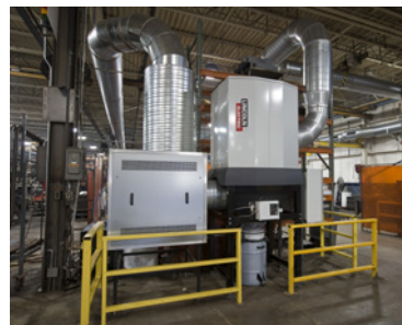
Push/Pull System installed at Elgin Sweeper Company
