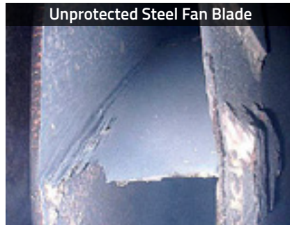
Unprotected steel fan blades are worn and must be replaced after 2-4 months of service.
