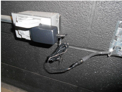
12V Power Supply Connection
