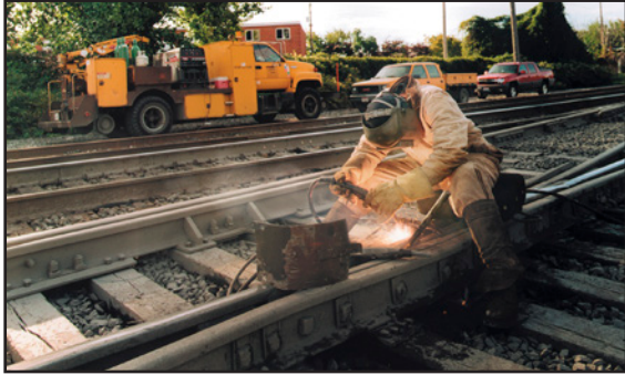
Railroad welding teams will appreciate the sizable air compressor, welding and 3-phase 240V power for grinders.
