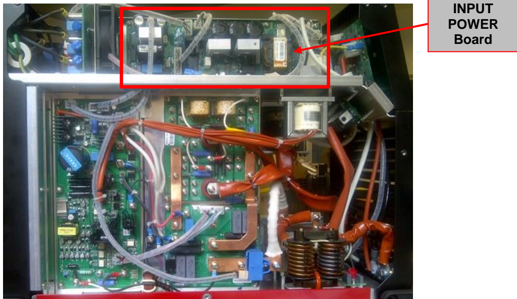
Figure 6 – W05X1461 INPUT POWER Board location
